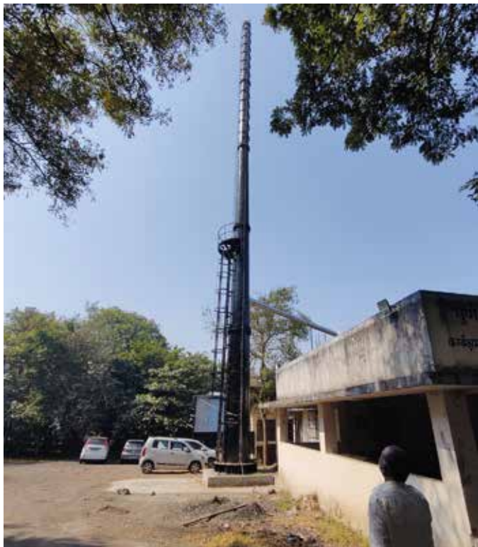
APC Chimney of 30 metres height as quoted by the attendant
